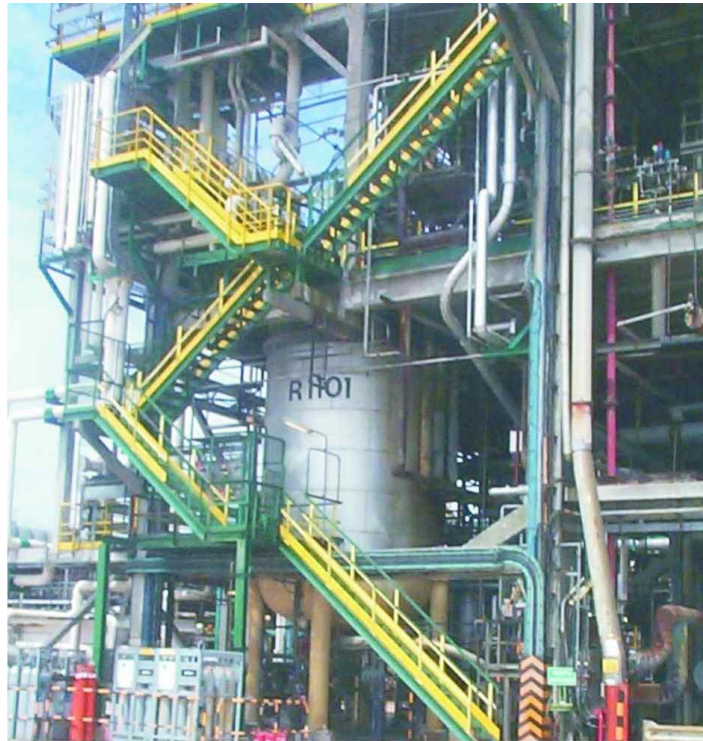
Figure 10 A CSTR reactor, used to make poly(ethene) in bulk.
